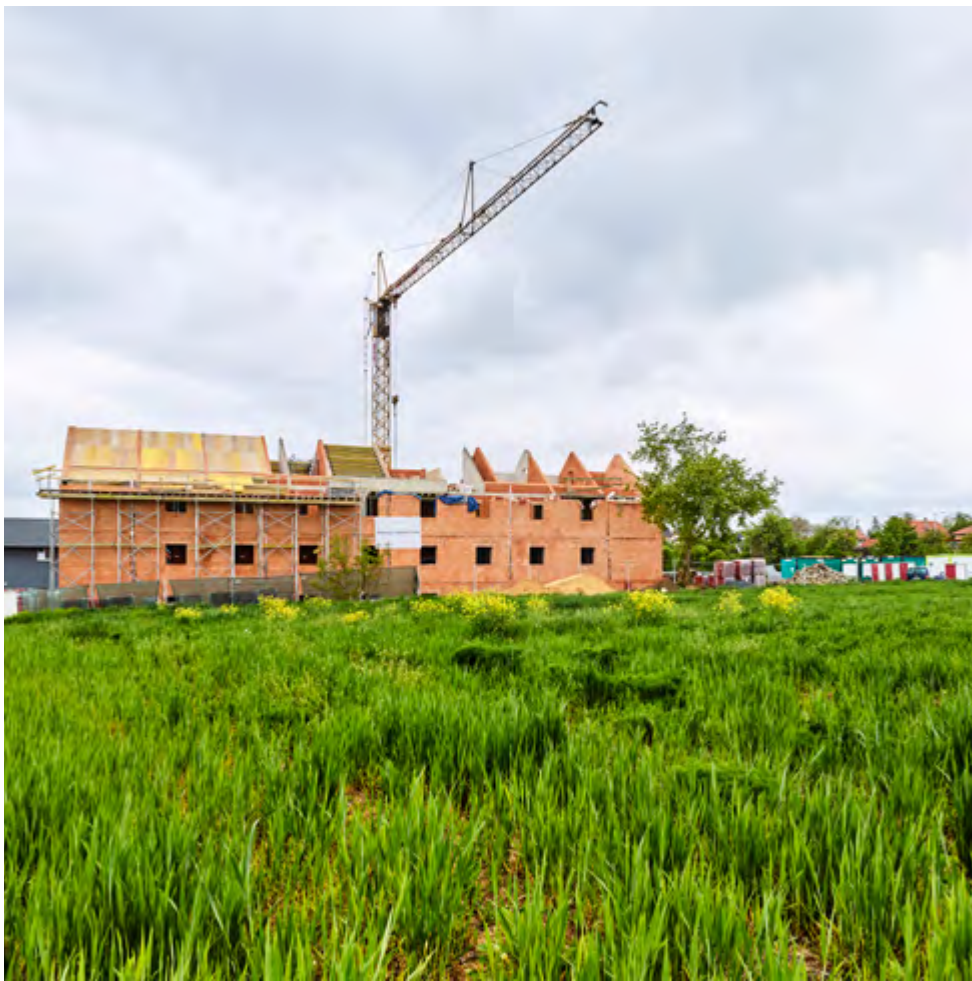
The Slivenec project, which features very uncommon concrete trusses, is a general delivery for Winning PS.
