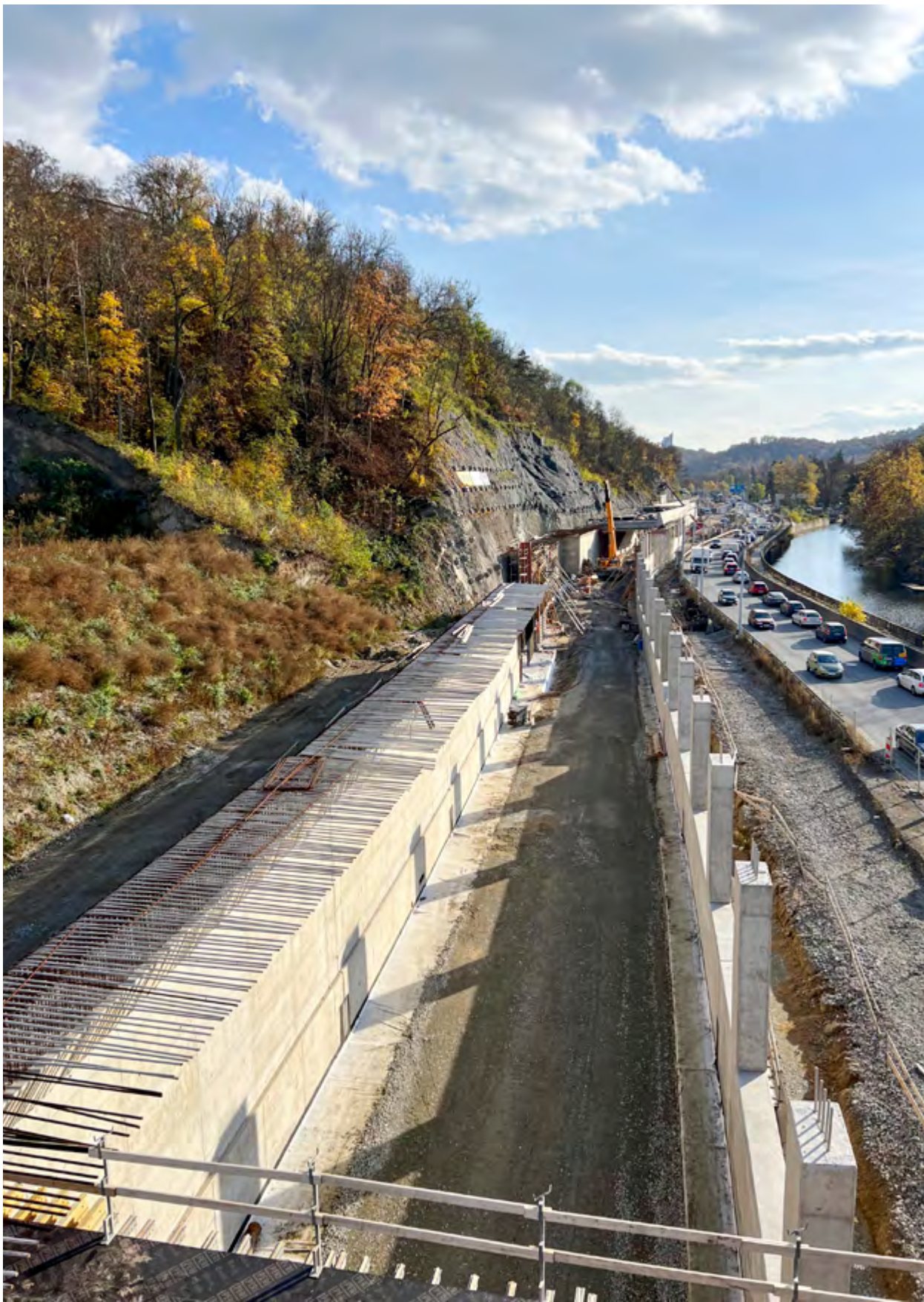
The large Brno ring road has a new 350 m long section leading from Královo Pole towards the exhibition centre. Reinforced concrete structures were supplied for it by Winning PS Pamstav. The two-lane gallery with one column, which is 7 metres in height, consists of 20 expansion units. Construction took a year and a half.
